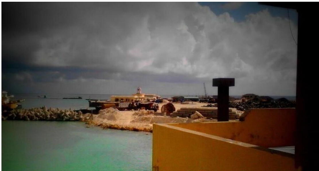
The breakwater of the harbor on West Reef was built by precast concrete caisson and accropode blocks to dissipate waves and prevent scour. Photo: nhjd.net
